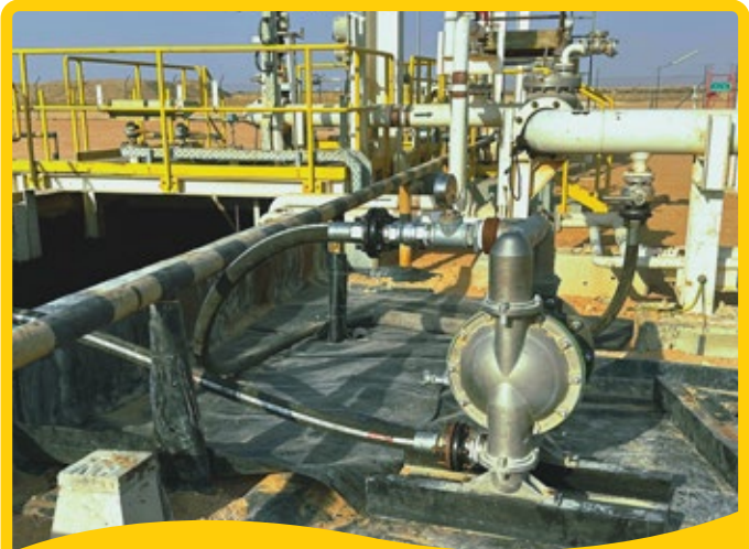
MWY - OIL PUMPING TO HIGH PRESSURE LINE
