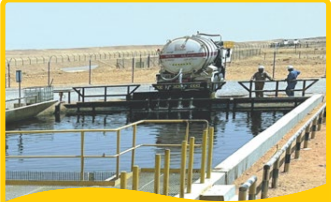
MWY - OIL PUMPING TO HIGH PRESSURE LINE
