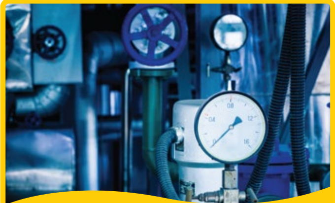
GAUGE TANK WITH HEATERS
