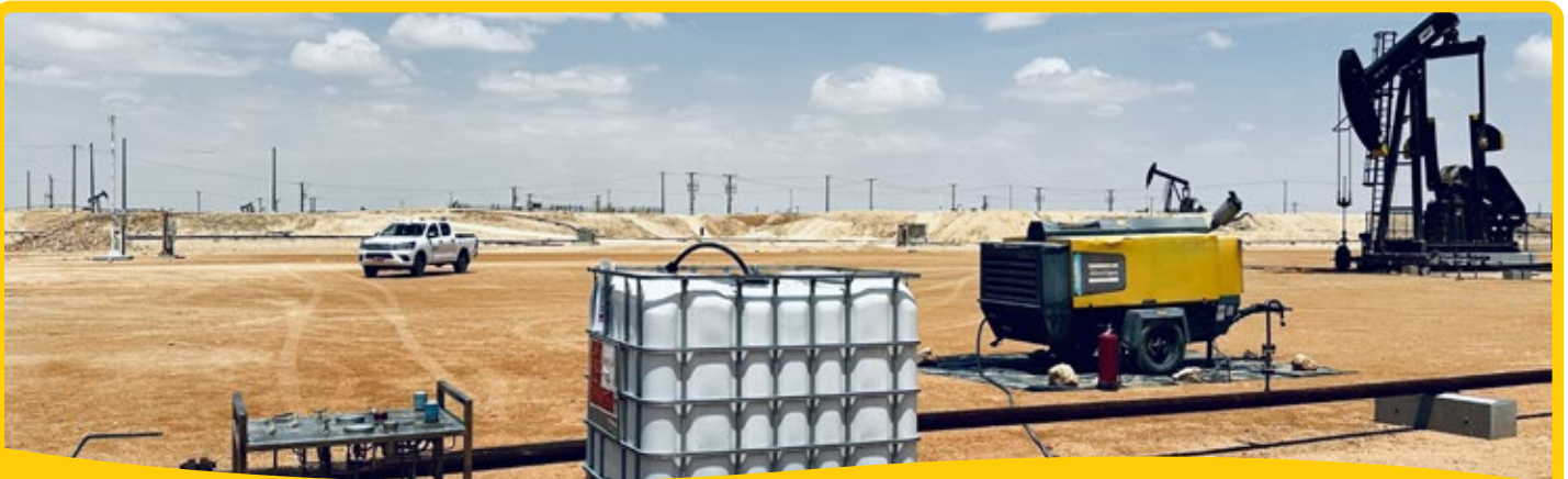
CHEMICAL INJECTION AT WELL FLOW LINE
